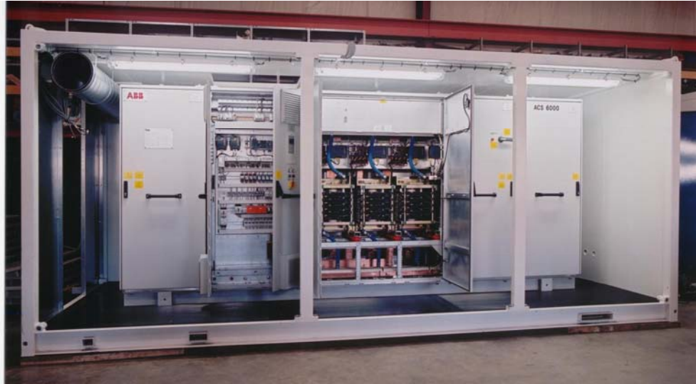
Fig 23 – Standalone 9MVA MV PWM VFD for dredger pump application (Bakker Sliedrecht)
